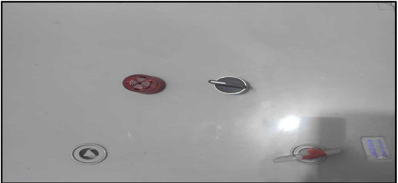
Fig 7 Electric Switch and Electric Buzzer
